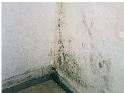
Example of degradation on a wall.
