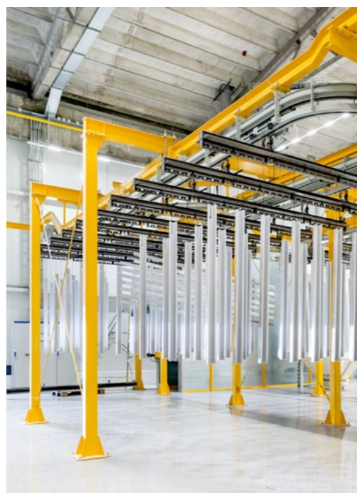
Modern solvent-free powder coating system with low water and energy consumption, pre-treatment tunnel with passivation (corrosion protection), and automated powder application with a recovery system.
